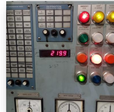
Old Electrical Control Panels
